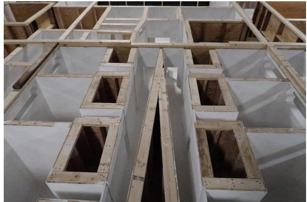
Headcell Influent Channel
