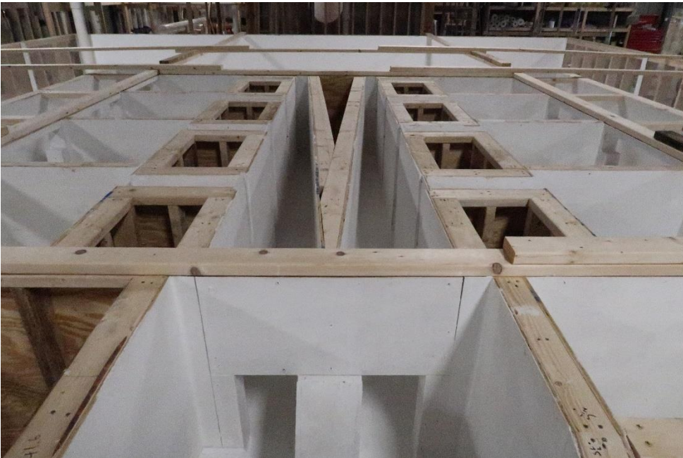
Headcell Influent Channel Isolation Gates
