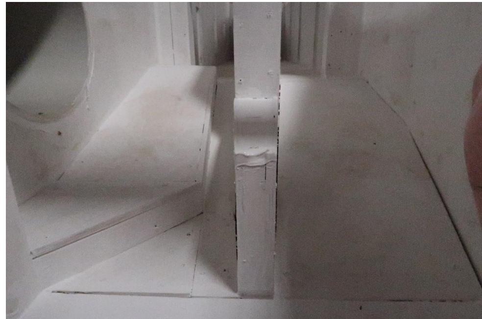
Influent Splitter Box
