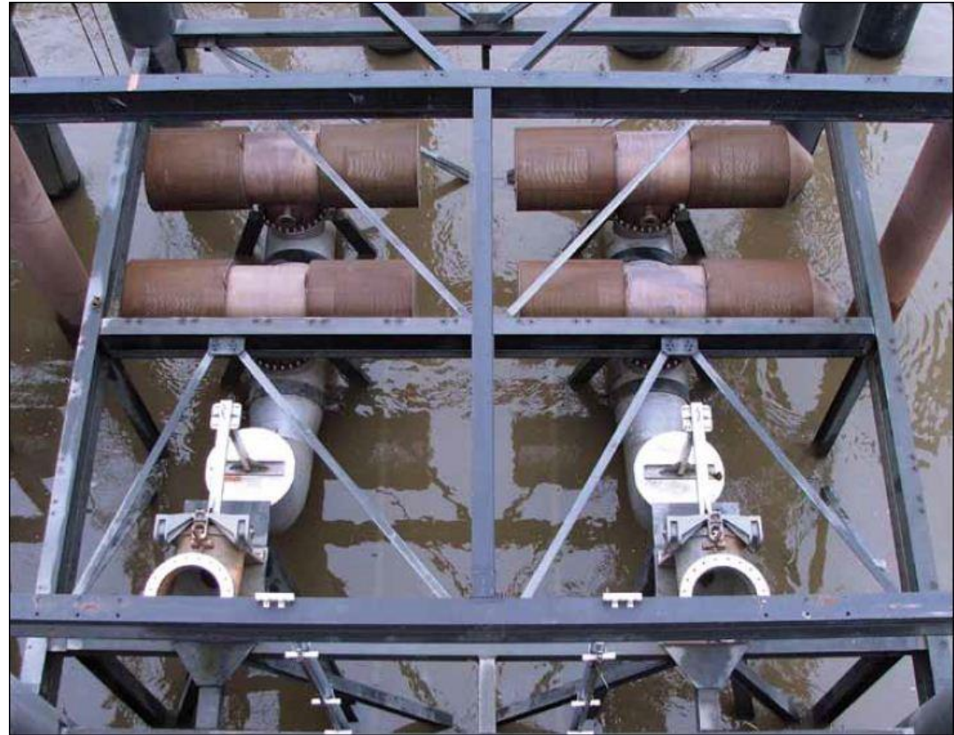
Desalination Plant Intake - Beckton, U.K.
